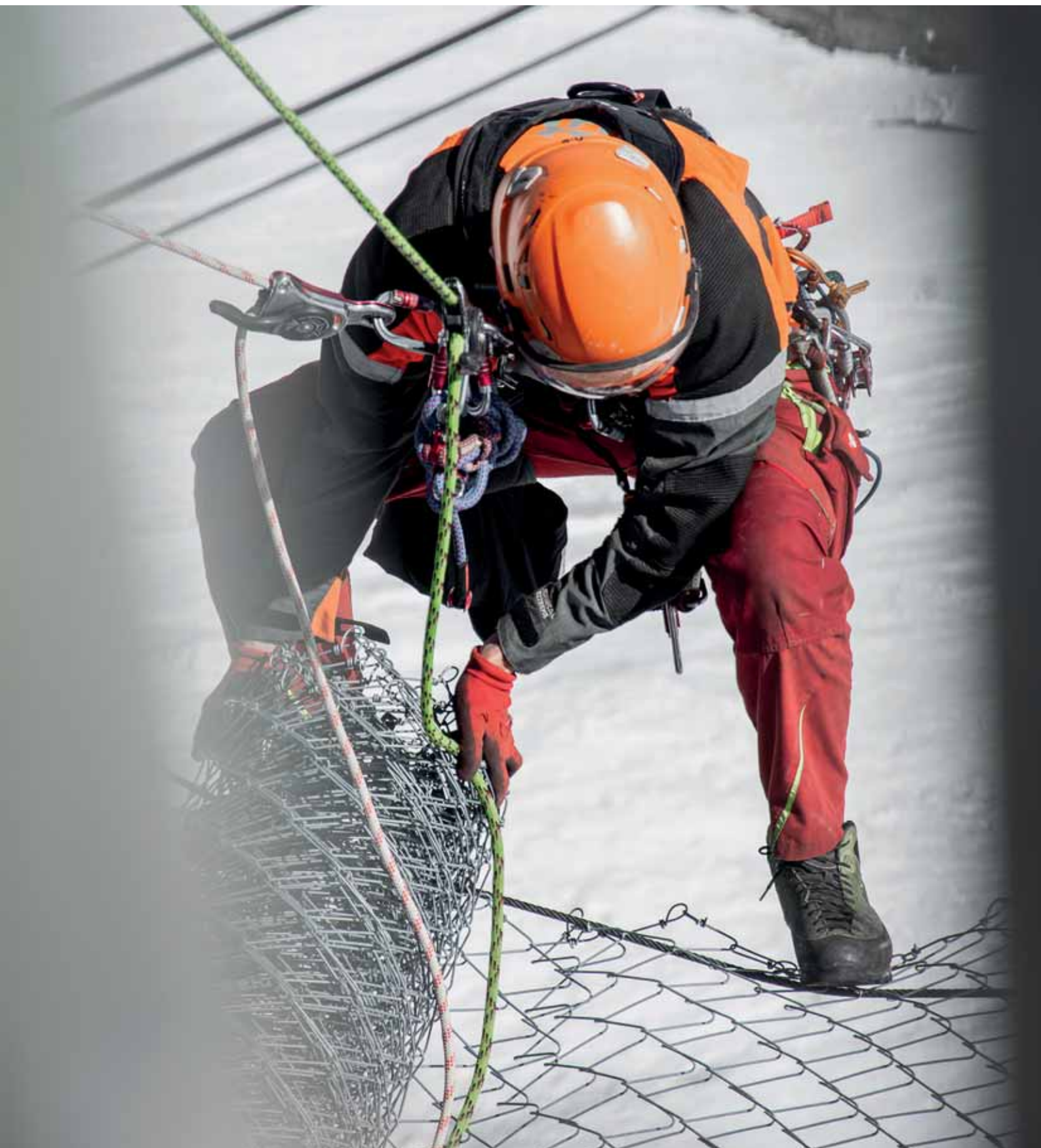
Installation of anchor points and safety nets for the reconstruction of the famous "La Botta" restaurant at Glacier 3000. Instalación de anclajes y redes para la reconstrucción del famoso restaurante «La Botta» en Glacier 3000. Les Diablerets, Switzerland (courtesy of Corde-Access SA, riggers Andrea Giazzi & Julien Guisolan, ph. Ari Cretton).
