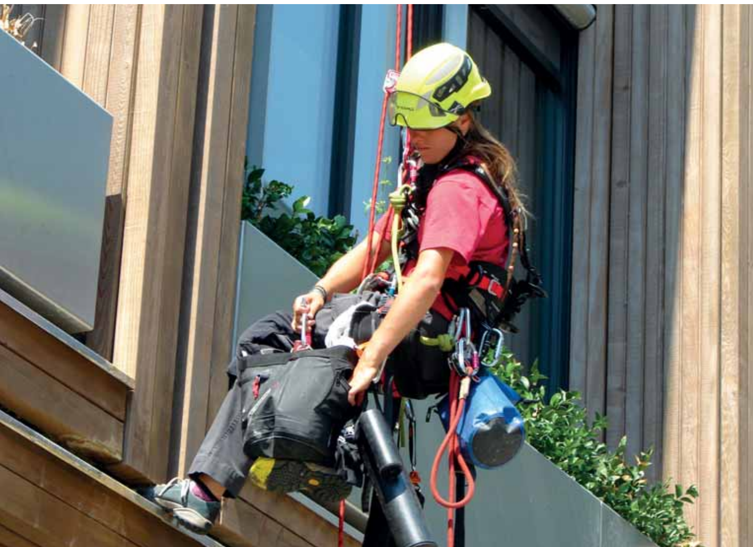
Gutter modification for a new building in Geneva (MSF). Modificación de los flujos de agua para el nuevo edificio en Ginebra (MSF). Genève, Switzerland (courtesy of Corde-Access SA, rigger Jenna Piron, ph. Corde-Access SA).
